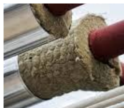
anomalous heat losses
