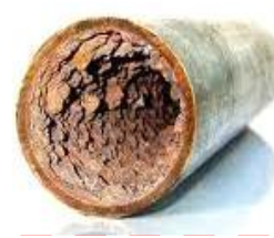
anomalous pressure losses
