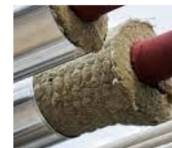
anomalous heat losses
